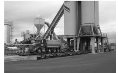
The Salem Blacktop and Asphalt Paving plant earns compliments for being a good neighbor with high standards
