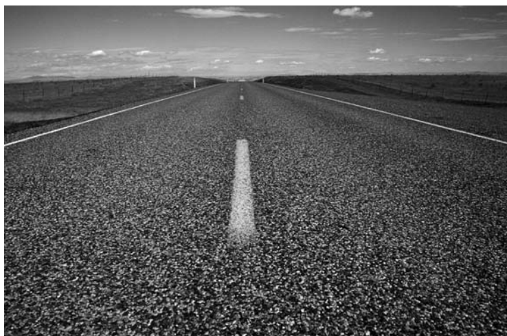
For roads that go on and on, achieving optimum density is critical to minimizing air and water infiltration, and the damage that results
