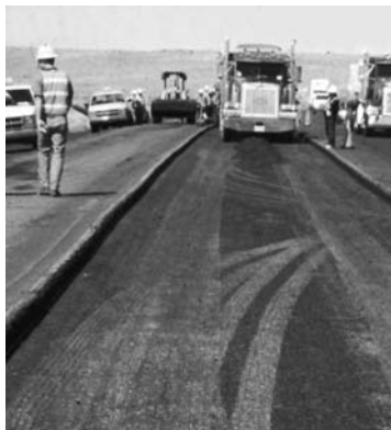
Haul trucks running over the tack coat before it has set will pick up the material and eliminate its bonding capability
