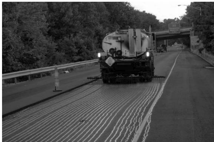
Blocked nozzles and non-uniform application of tack coat will result in a poor bond between the existing surface and the new asphalt layer
