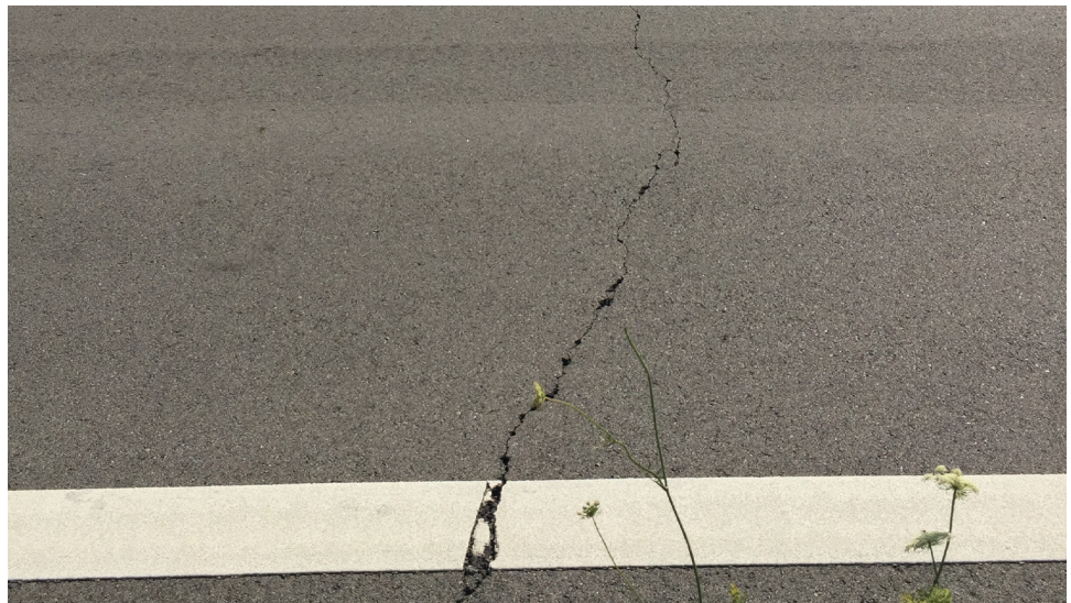
Figure 12. Transverse crack with adjacent deterioration
