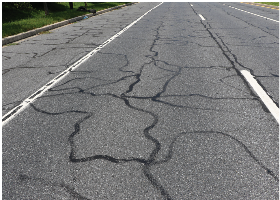
Figure 8. Heavy block cracking with sealed cracks
