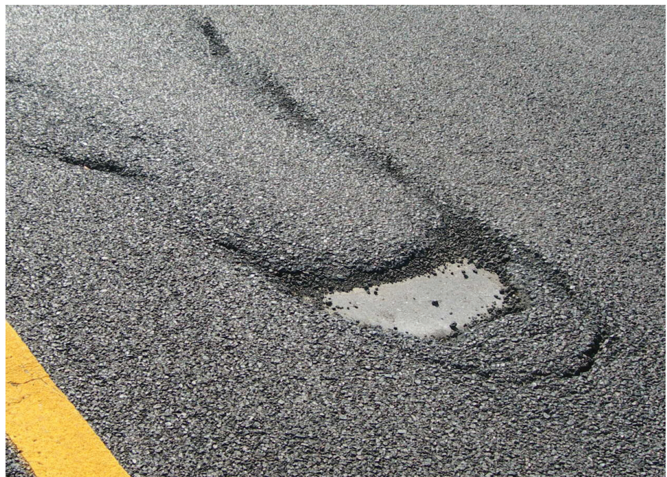
Figure 20. Slippage close up
