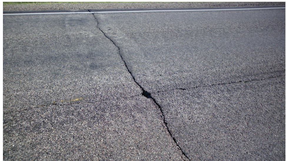
Figure 13. Transverse crack with adjacent snowplow damage
