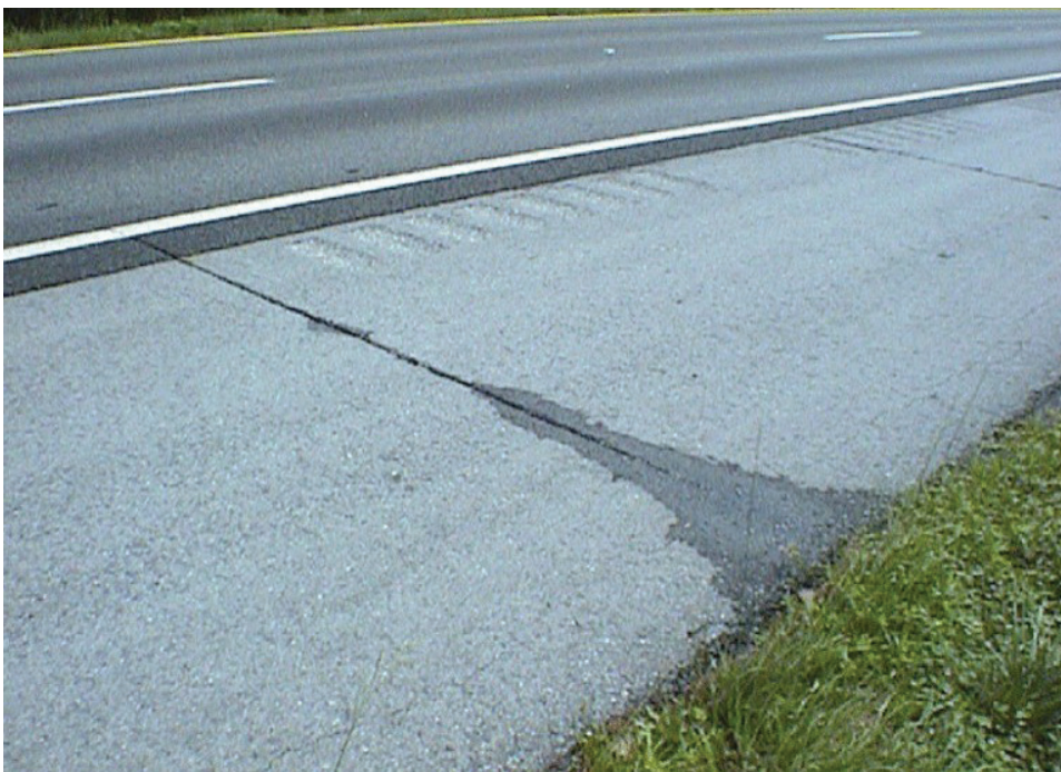
Figure 22. Water penetration in a pavement
