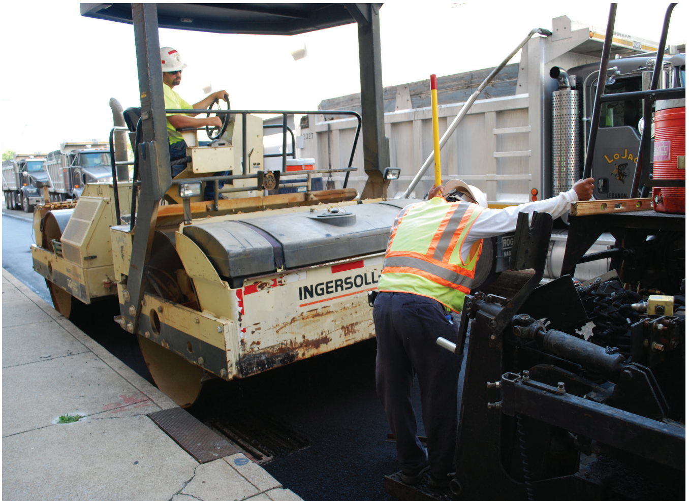
A compactor closely follows the paver on a demonstration Thinlay project in Nashville.
