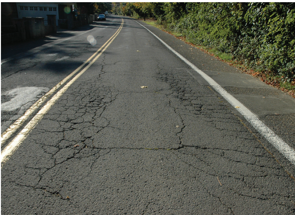
Figure 10. Extensive alligator cracking
