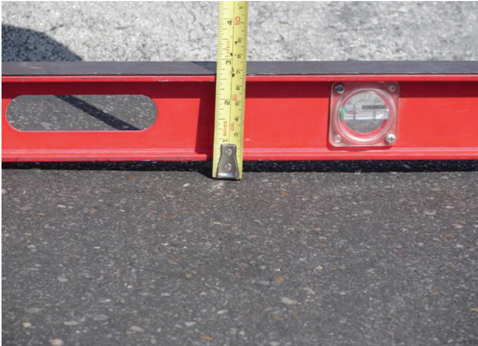
Figure 6. Rut depth less than \frac{1}{2} inch
