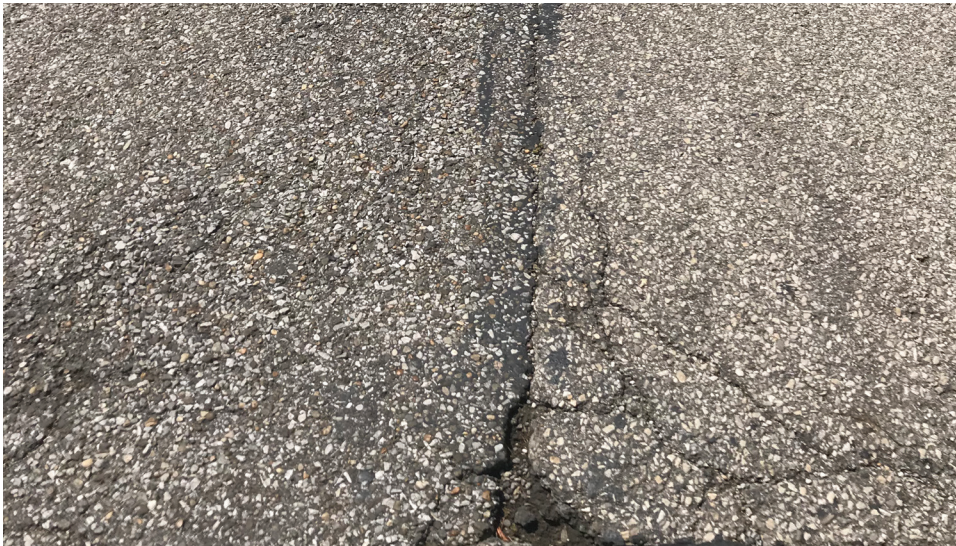
Figure 17. Slight raveling in and adjacent to longitudinal crack
