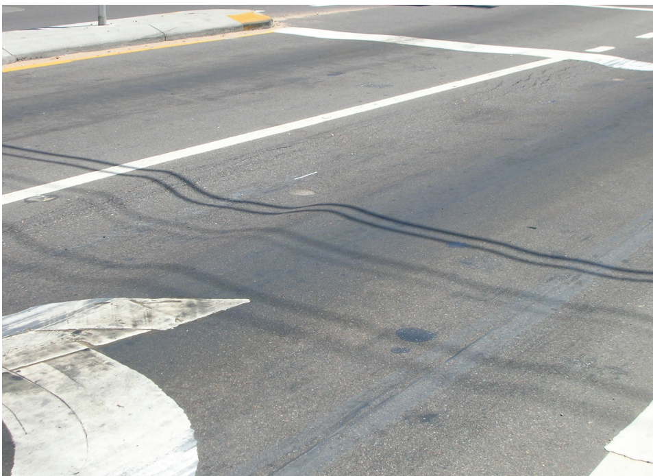
Figure 7. Rut depths exceeding 1 inch
