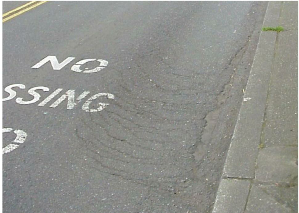
Figure 19. Asphalt pavement slippage
