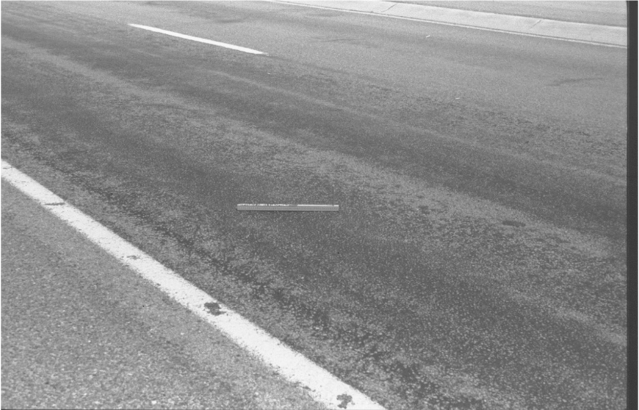
Figure B.1 Bleeding/Flushing Surface
