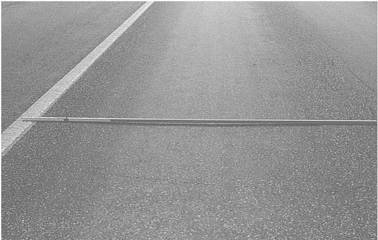
Figure B.19 Rutting – Load Associated
