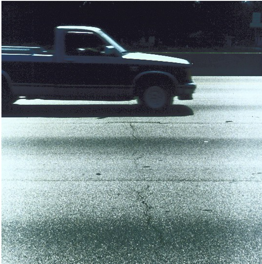
Figure B.11 Reflection Cracking – Narrow Cracks
