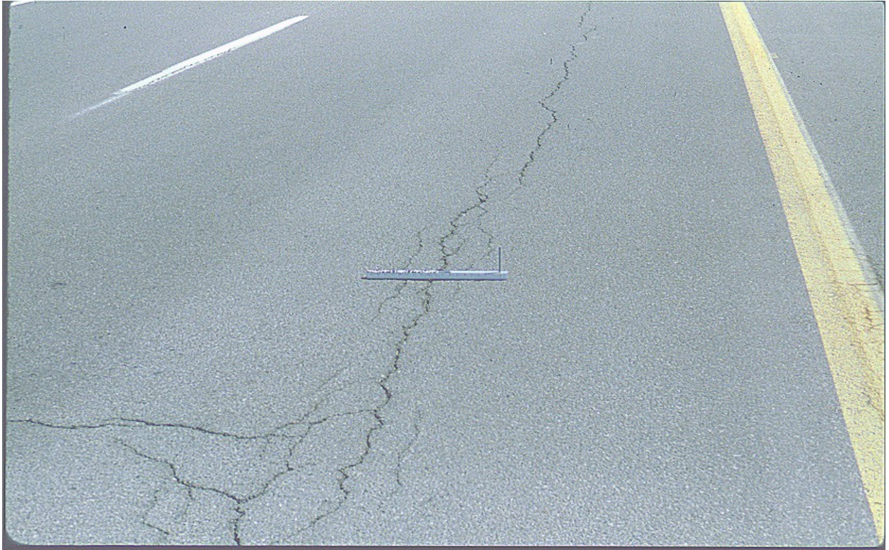
Figure B.7 Longitudinal Crack - Low
