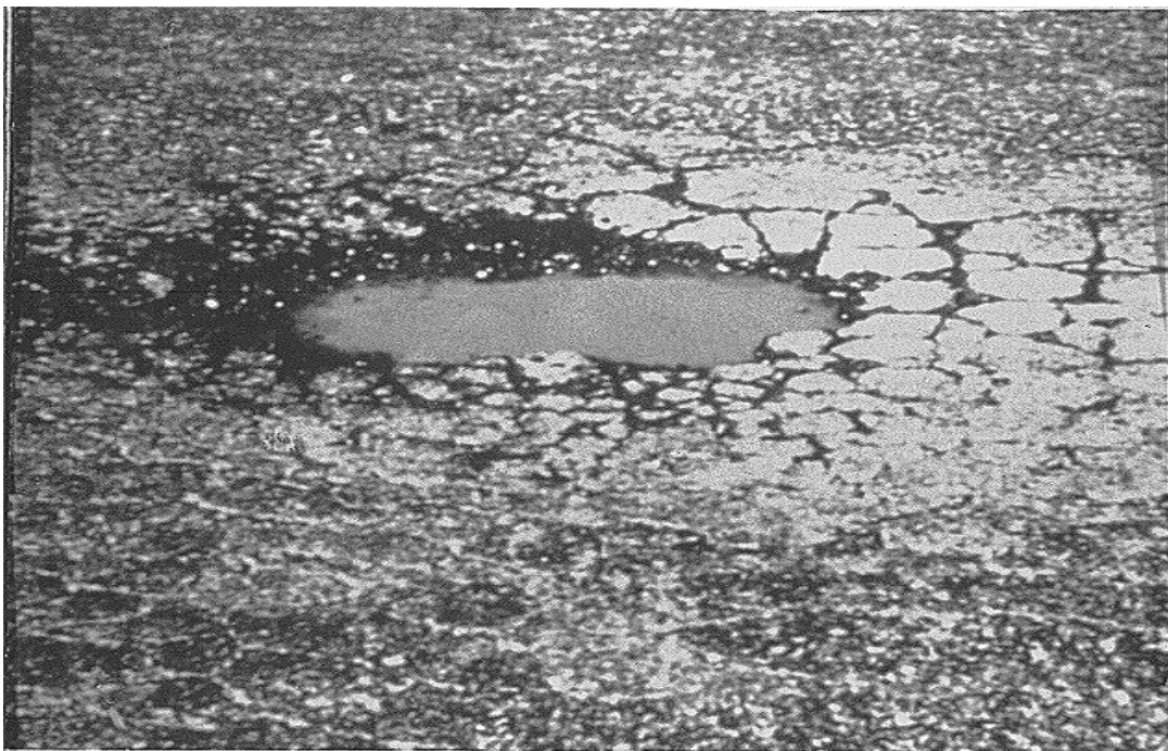
Figure B.16 Potholes
