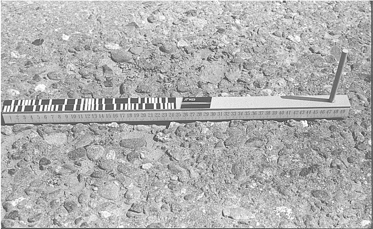
Figure B.17 Raveling
