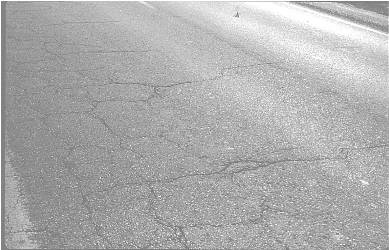
B.10 Random Cracking - Moderate Cracks
