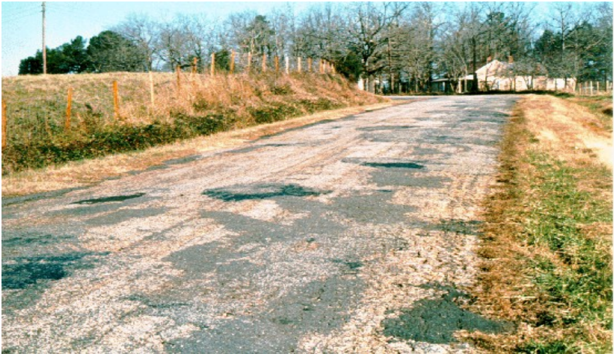
Figure B.18 Disintegrated Surface
