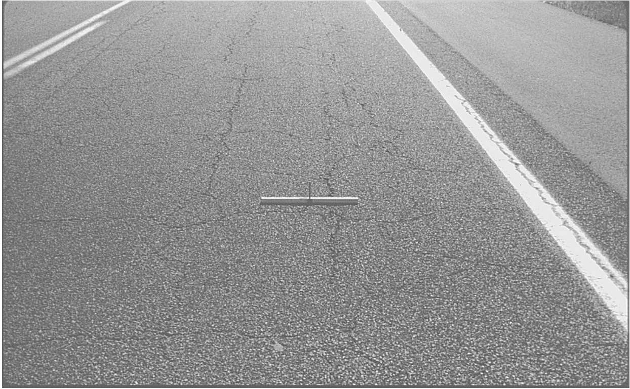
Figure B.9 Random Cracking – Narrow Cracks
