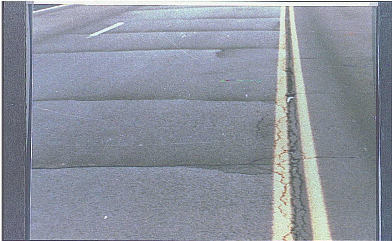
Figure B. 12 Reflection Cracking—Wide Cracks
