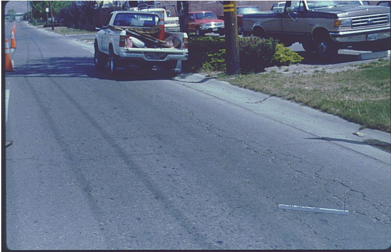
Figure B.3 Alligator Cracking – Low
