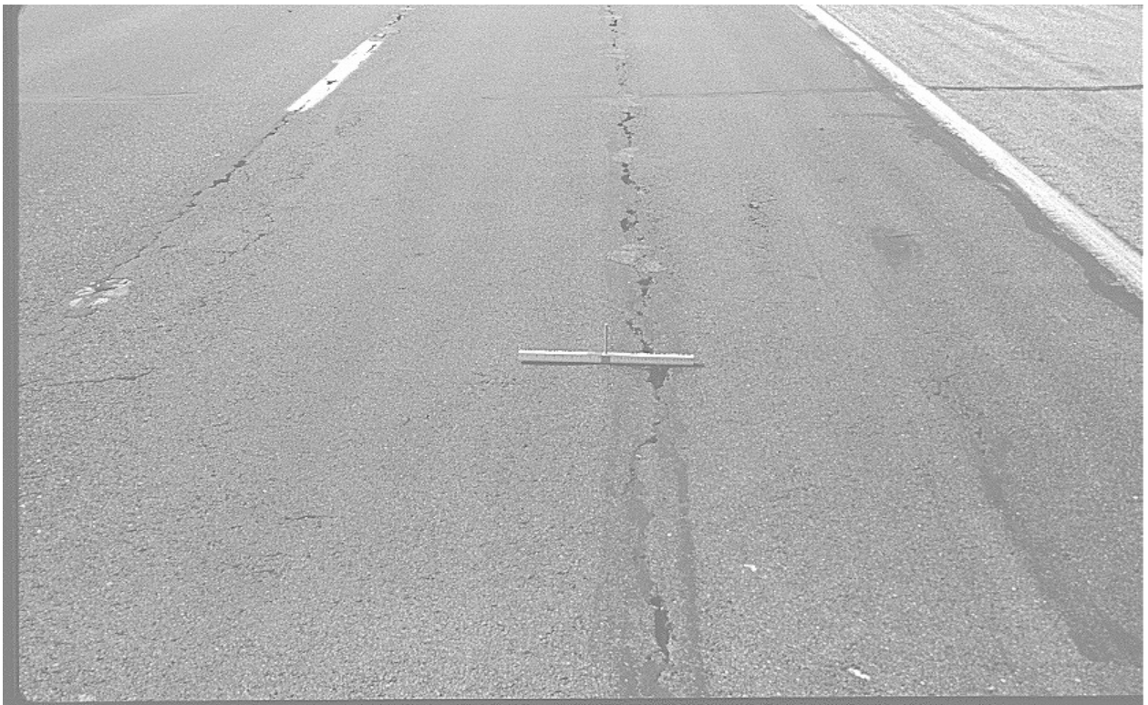
Figure B. 8 Longitudinal Joint—Moderate
