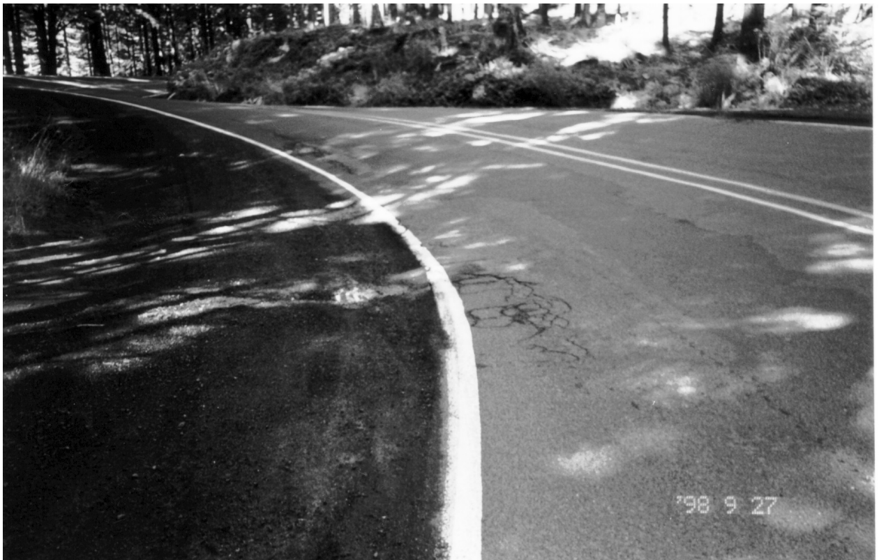
Figure B.6 Edge Cracking with Distortion
