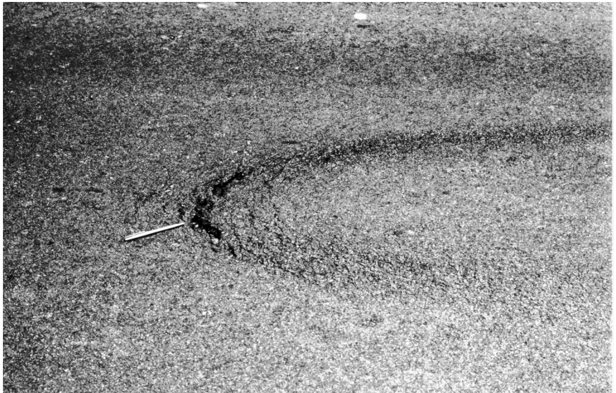
Figure B.14 Slippage Cracking
