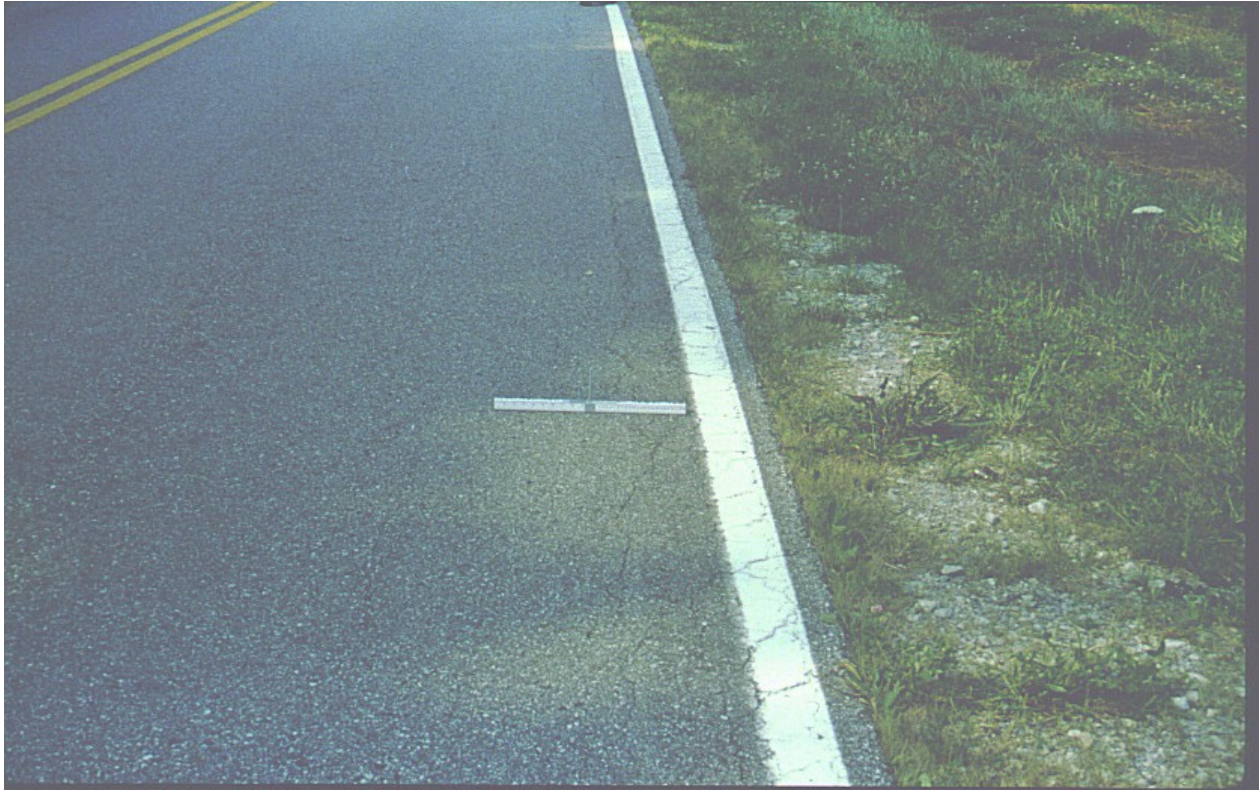
Figure B.5 Edge Cracking without Surface Distortion
