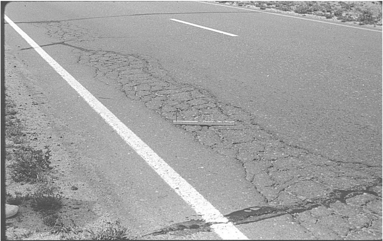
Figure B.4 Alligator Cracking - Moderate
